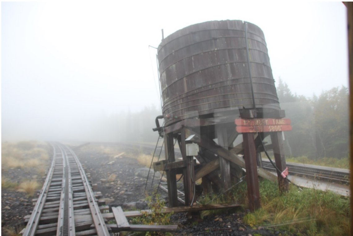
The water tank may look like it is crooked, but it is dead level.
