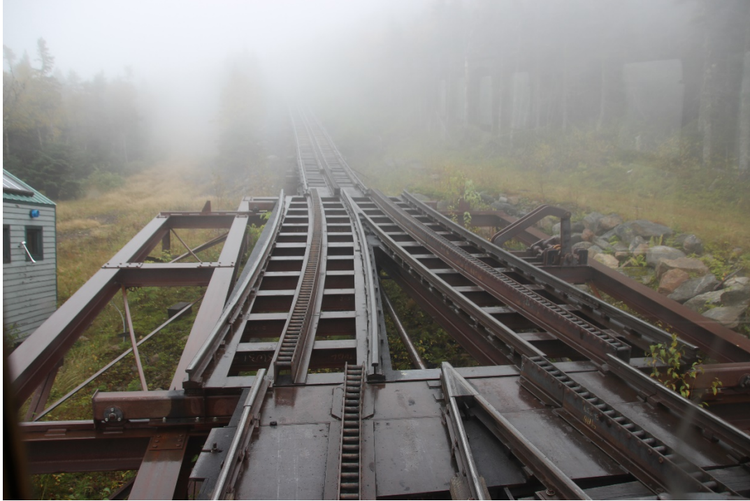
The upper hydraulic switch in the the passing track is seen swinging into place. The solar panel power house is to the right.
